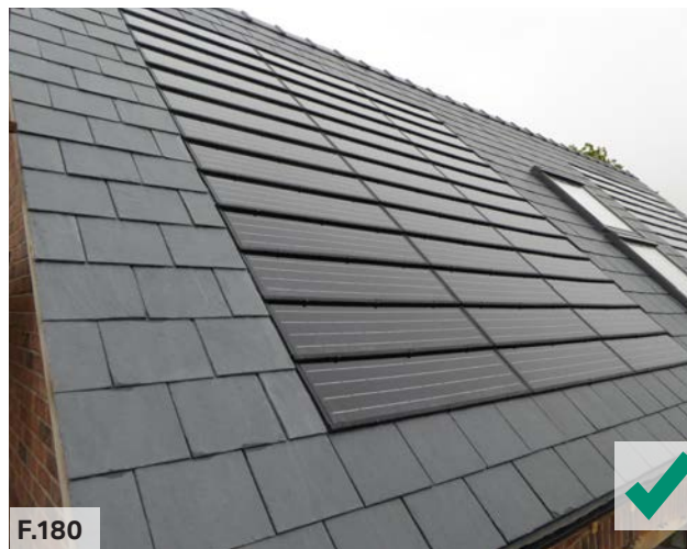
Figure 180: Integrated solar panels on slate roof.
